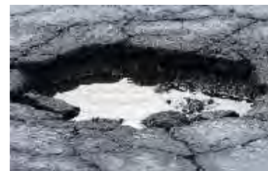
Fig.1. Condition of roads with potholes.
